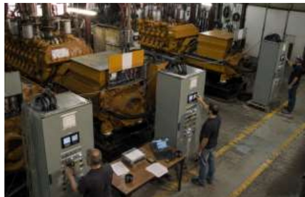
Figure 2: Reliable Load Bank Testing
