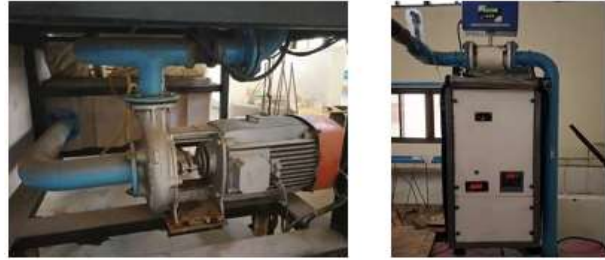
Fig. 5. Electric motor and electromagnetic flow meter with panel
