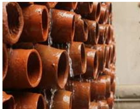
Fig. 4. CoolAnt Beehive cooling installation, a sustainable air-cooling solution developed by Ant Studio.
