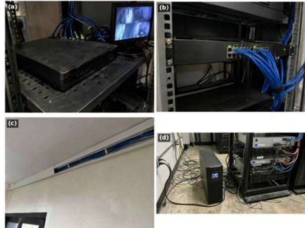
Figure 3. Installed hardware: (a) 8-channel DVR with live-view monitor; (b) rack-mounted network switch with Cat6 patching; (c) cable trunking; (d) UPS beside the equipment rack.
